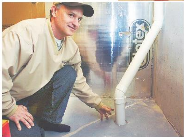
David Holmes, a radon specialist, points out the radon mitigation system piping installed in the Cagwins' basement. The EPA recommends all homeowners conduct a short-term radon test.
